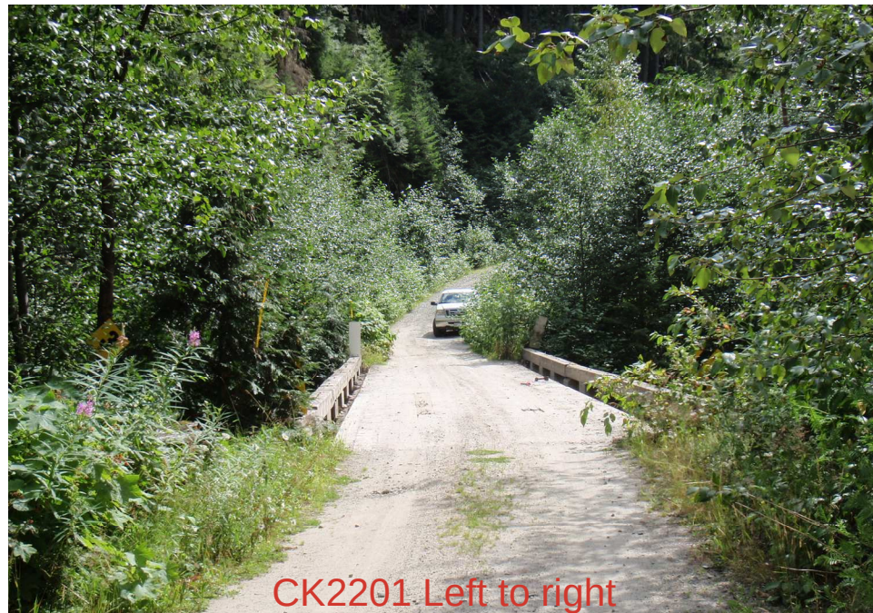
CK2201 Damage deck 4
